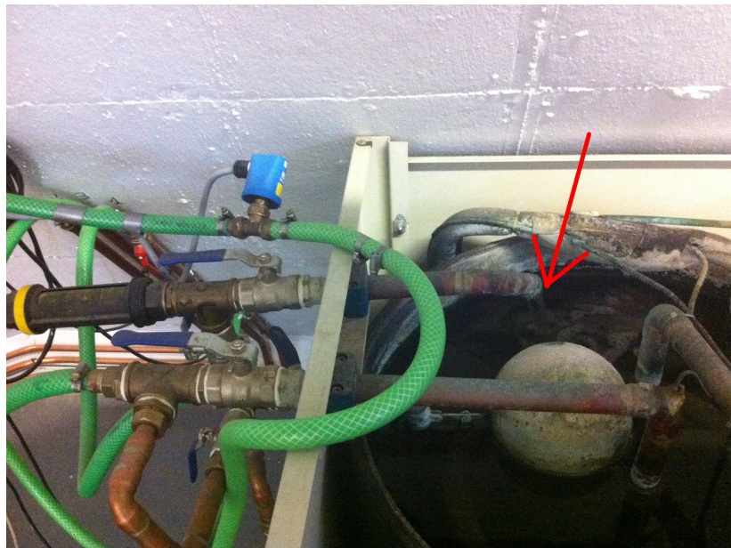
Picture 10: the water cooling system.
